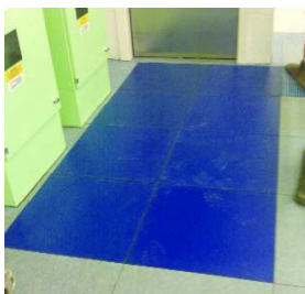
ITDecom Tiles installed in Royal Bank of Scotland Data Centre.
